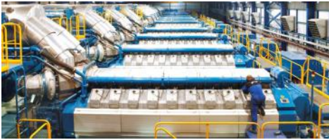
Typical configuration shown for interior of Wartsila power plants
