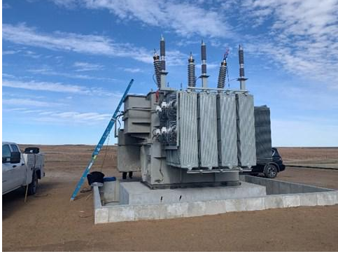
New transformer set at Kingman/Cunningham site
