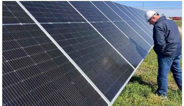
Above: KPP Board Member Chris Komarek (Ellinwood) inspects the bifacial solar panels at the new Fredonia Solar Farm.
