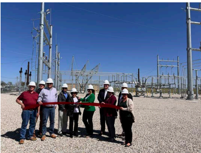
Above: Winfield Tie Switchyard ribbon cutting included dignitaries from the Kansas Legislature, Winfield City Commission, Winfield City Staff and GridLiance.
