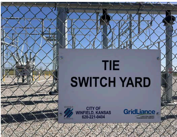
Above: New Tie Switchyard constructed by the City of Winfield and GridLiance.
