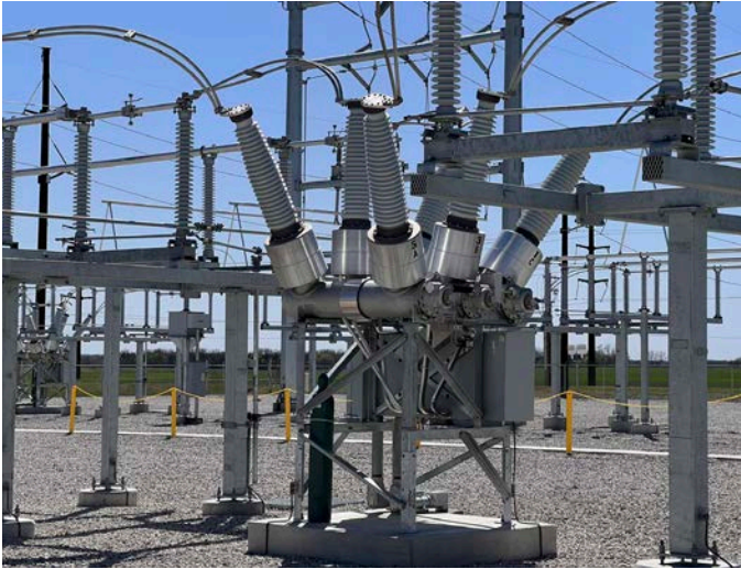
Above: 138-kilovolt (kV) breaker inside the new Tie Switchyard. The breaker is currently operating at 69 kV.
