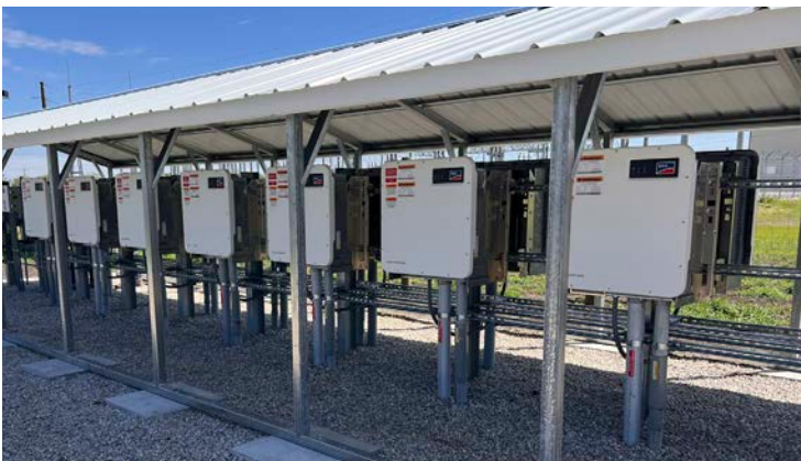
Above: A bank of inverters at the Fredonia Solar Farm.
